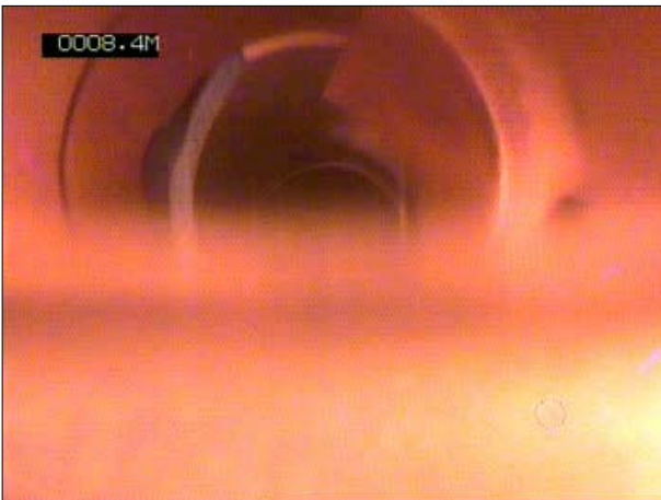
Photo: 114_6a 8.4m, Sewer Broken, from 12 to 12 o'clock
