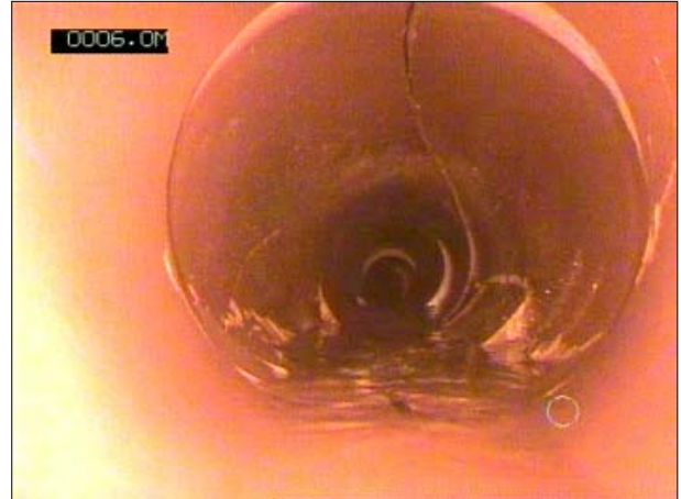
Photo: 112_4a 6m, Multiple Cracks, from 07 to 03 o'clock, Start
