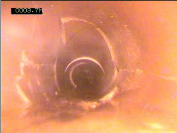
Photo: 109_1a 3.7m, Multiple Cracks, from 12 to 12 o'clock, Start
