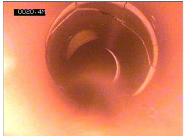
Photo: 116_8a 20.4m, Multiple Cracks, from 10 to 03 o'clock
